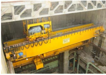
Figure 1. Overview of 280/85T EOT Crane in RCB.
